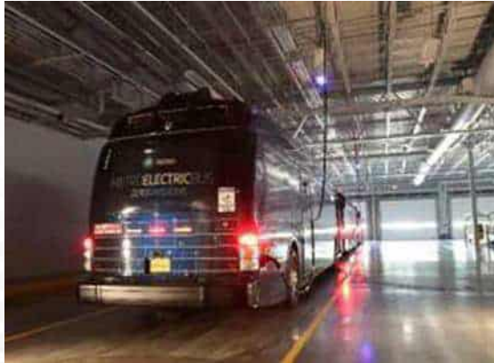
Bus Charging Area
