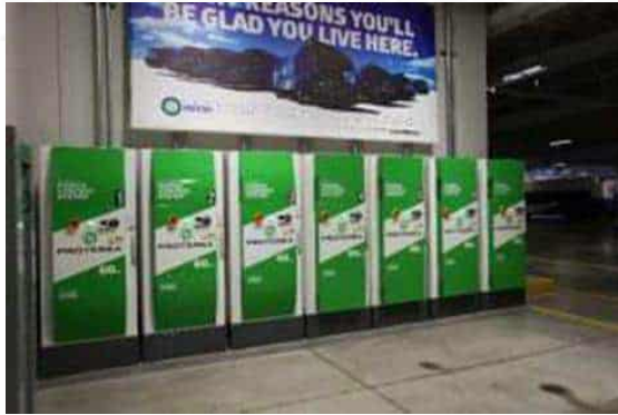
Existing Charging Stations
